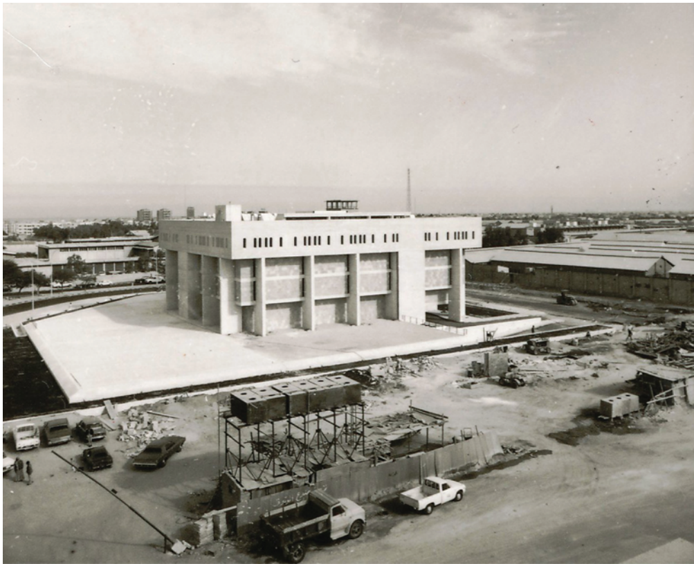
Kuwait Fund for Arab Economic Development, construction photo, c. 1972. Courtesy PACE Archives.
