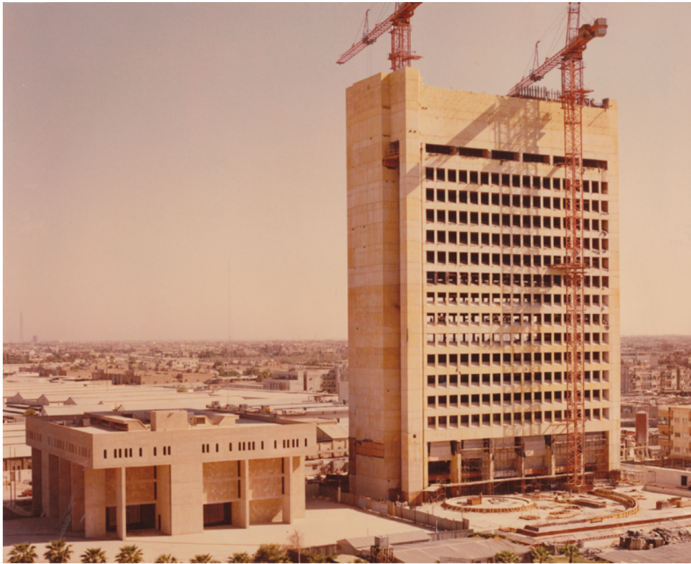
TAC with PACE, tower addition to Kuwait Fund for Arab Economic Development (1974–1981), construction photo. Courtesy PACE Archives.
