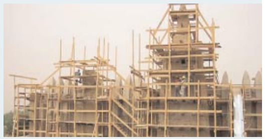
The completed scaffolding system along the east façade and central minaret. A chute, visible to the right of the minaret, was installed to facilitate the removal of debris from the roof of the mosque.
